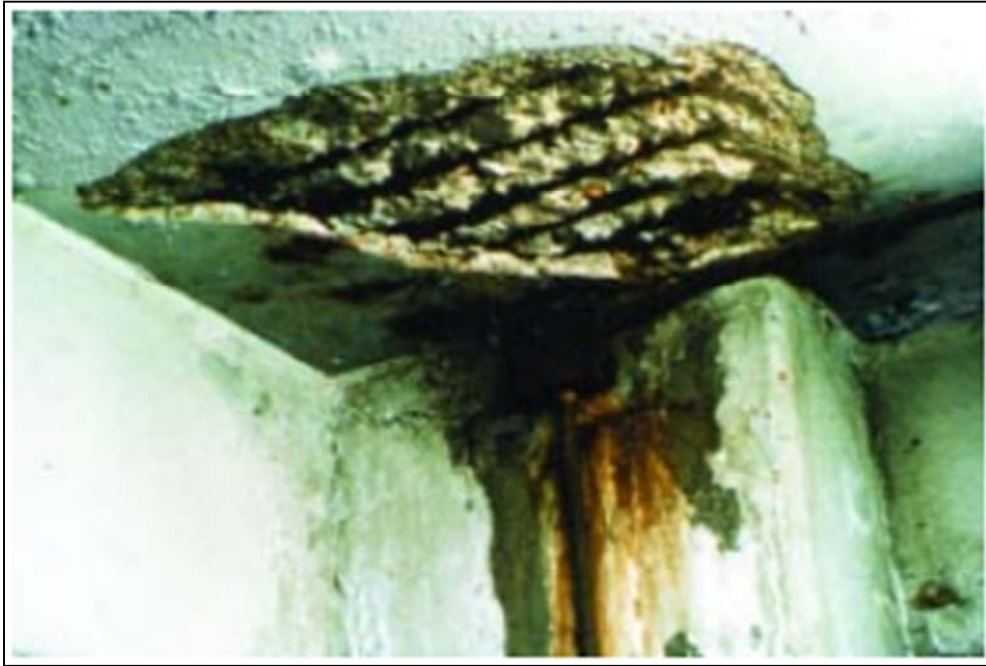
Figure 1. Corrosion of reinforcing steel is the most common cause of concrete deterioration [1].
